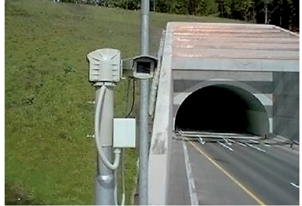
Optical Communications Traffic Control Systems.
